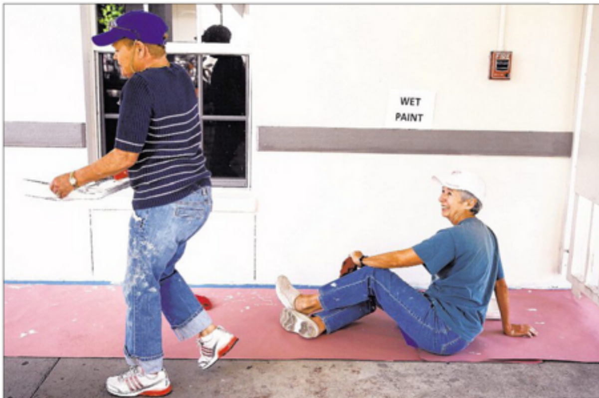
Greater Naples Leadership volunteers Vi Steffan, left, and Myra Williams, both of Naples, laugh Thursday while painting the outside walls at St. Matthew's House in Naples.
