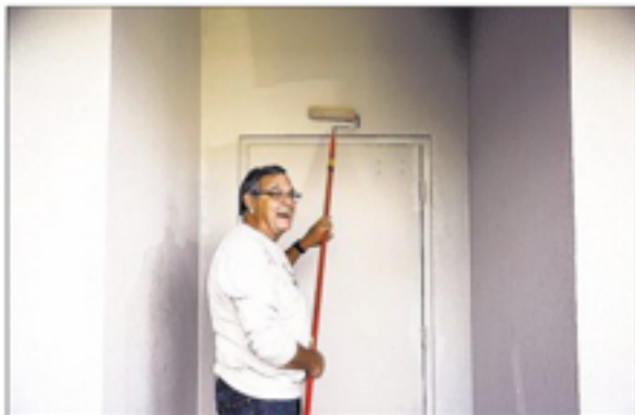
Greater Naples Leadership volunteer Ron Ferguson, of Naples, paints a wall Thursday at St. Matthew's House.
